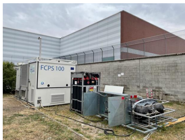
Figure 3 Example of test on site for EVERYWH2ERE Genset with bundles
